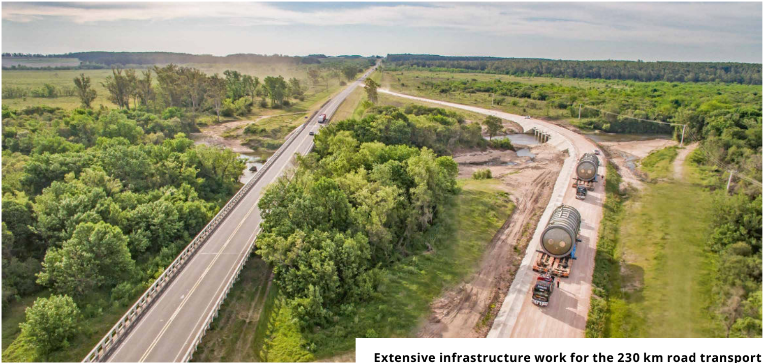
Extensive infrastructure work for the 230 km road transport in central Uruguay, incl. the building of 28 bypasses
