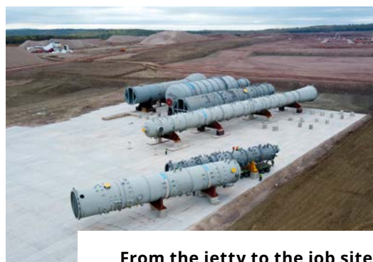
From the jetty to the job site: Overland transportation of the 81.7 m, 357 MT fractionator and further OSHL units
