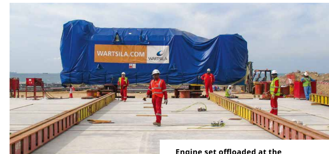
Engine set offloaded at the site near the foundation for final positioning
