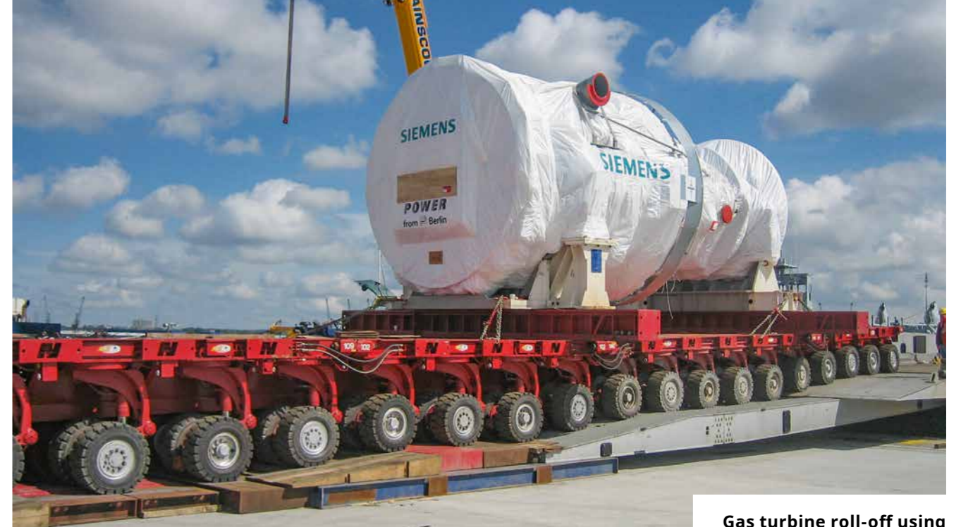
Gas turbine roll-off using an 18-axle, four-file SPMT over an extended ramp
