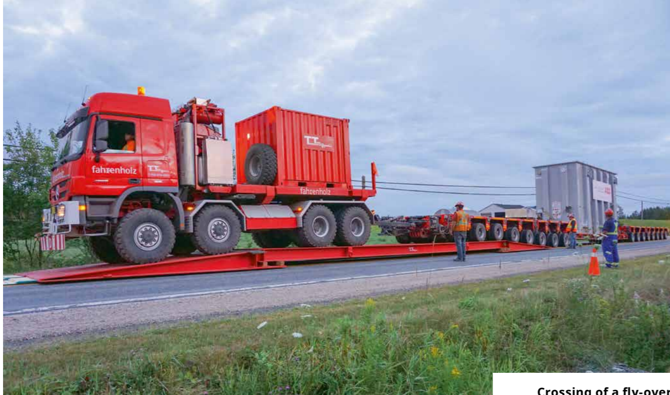
Crossing of a fly-over bridge that was installed to protect a culvert
